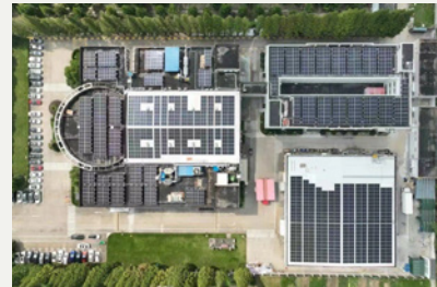
Solar panels at Kunshan, China Energy plant.
